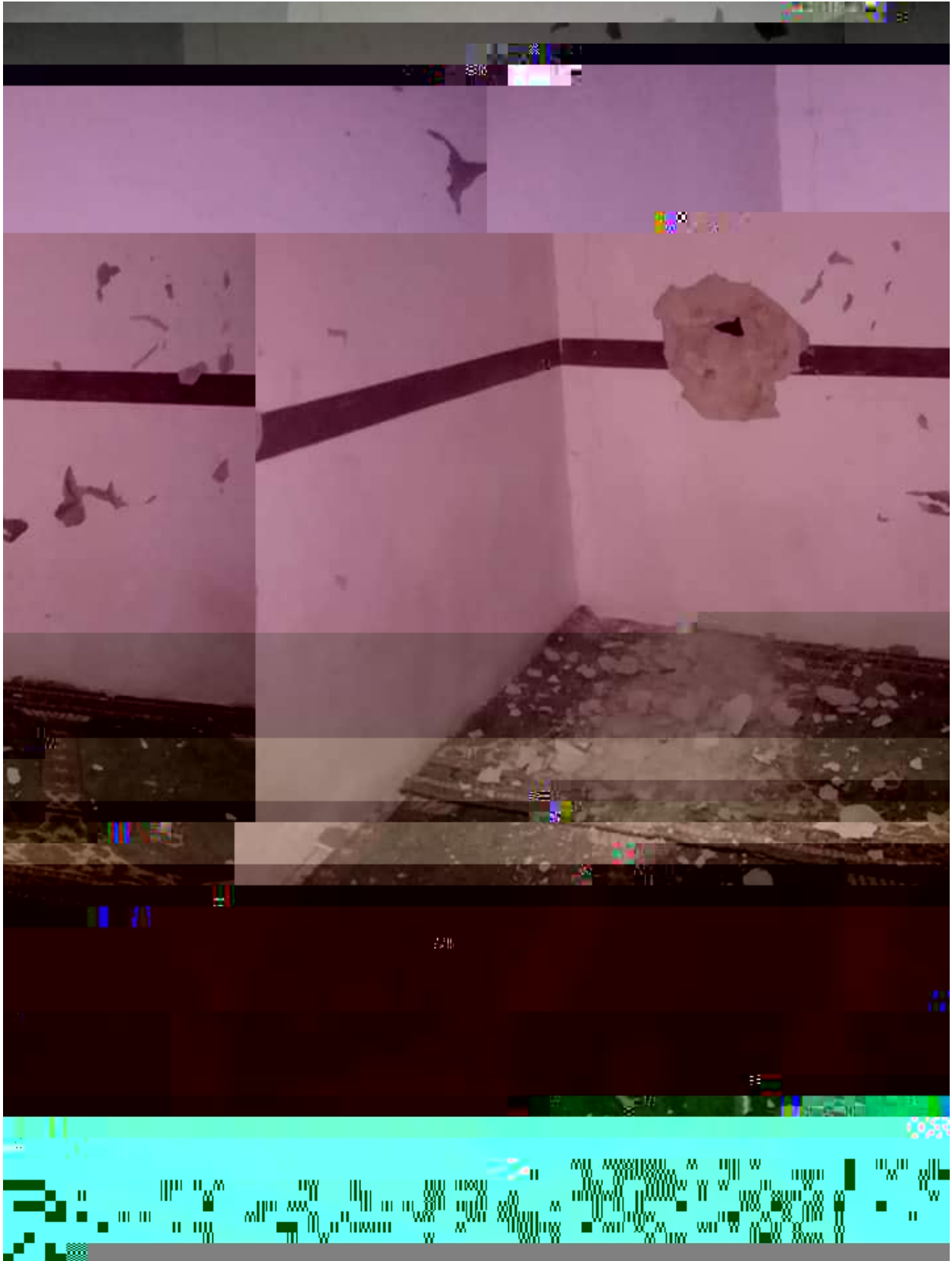
Damage to a wall in the mosque (Media Center in Talafah Village; November 20, 2018)
