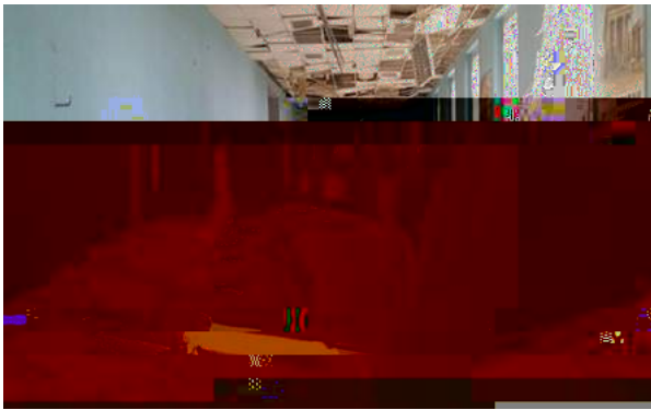
Figure 63. Damage inside gallery (posted by DGAM; March 28, 2016)
