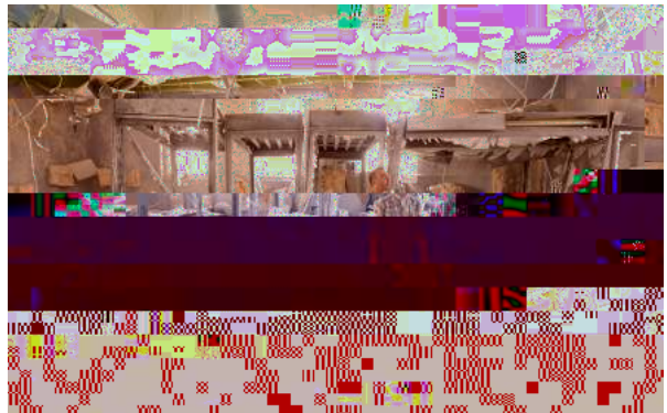
Figure 64. Damage inside gallery (Sputnik; March 28, 2016)
