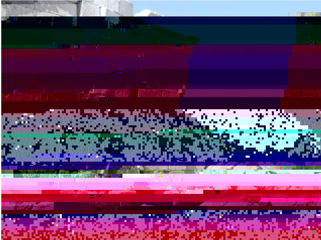
Severe damage to the walls.
