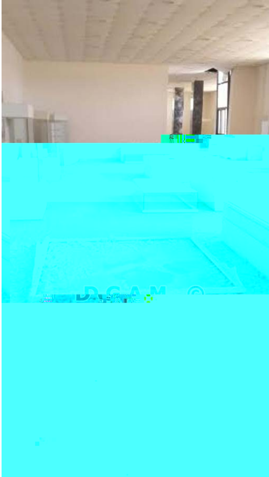
Museum of Daraa, interior damage (DGAM; July 3, 2015)
