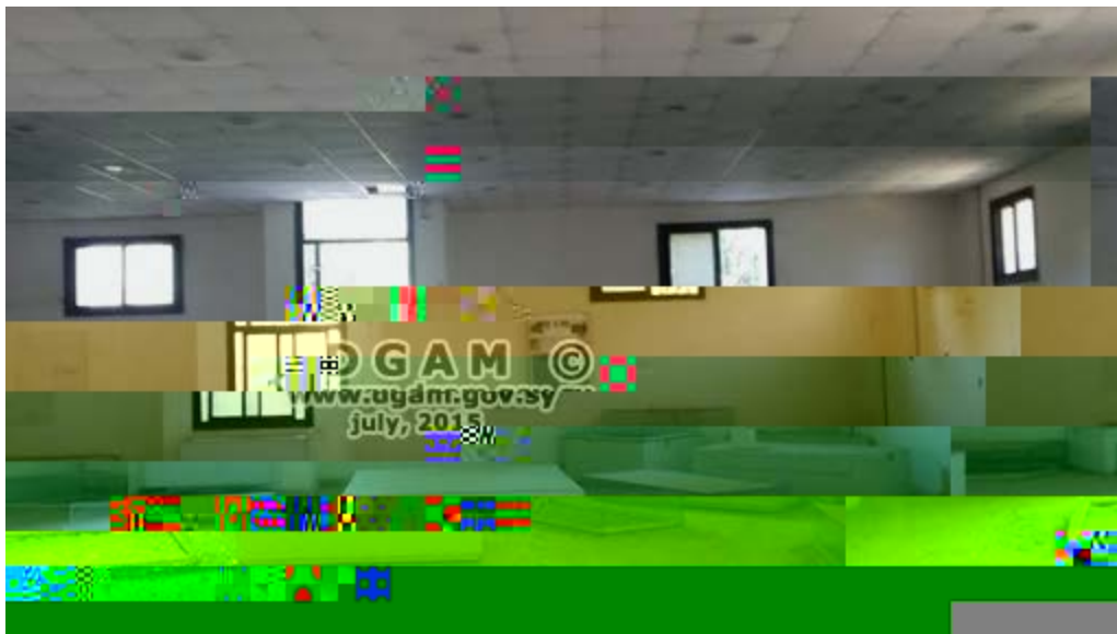
Museum of Daraa, interior damage (DGAM; July 3, 2015)
