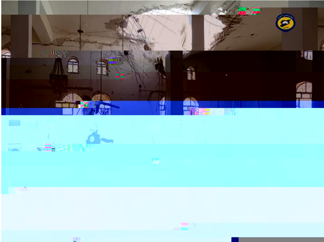
Damage to the interior of the Grand Tarmala Mosque (The White Helmets; October 20, 2016)
