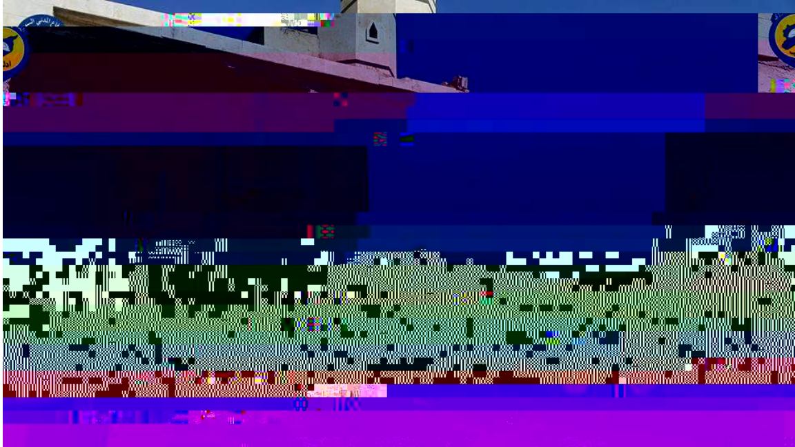
Damage to Abu Bakr al-Sadiq Mosque (The White Helmets; October 28, 2016)
