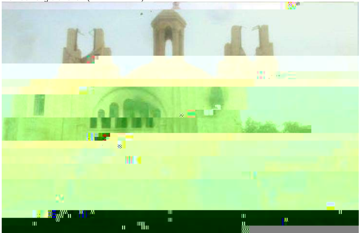
Fire damage and the removal of crosses at Mar Gewargis Church (Bartella Cafe; October 25, 2016)
