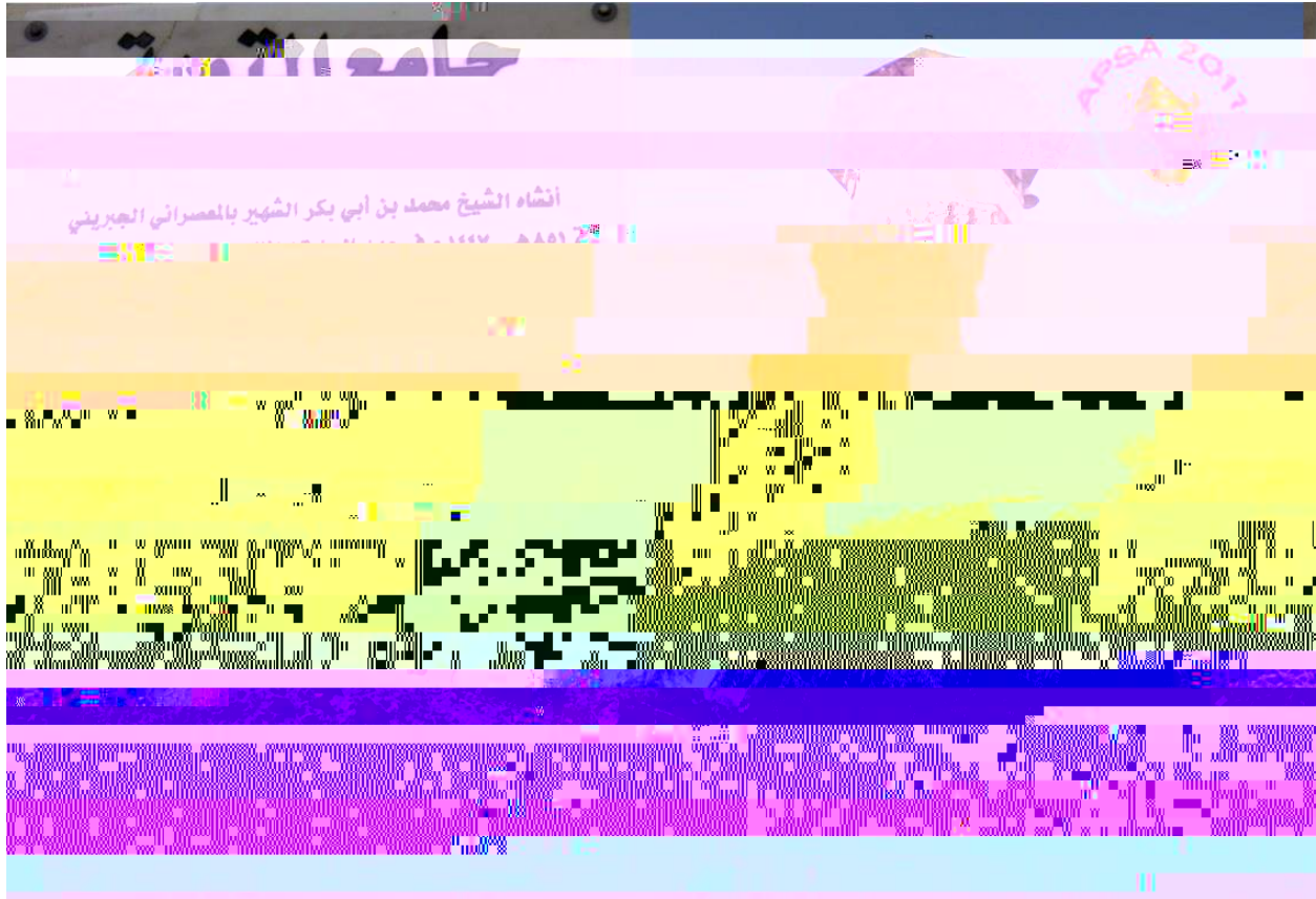
Damage to courtyard of al-Tawba Mosque (APSA; October 6, 2016)
