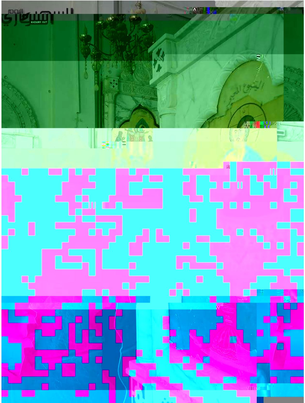
Damage to the interior of Saint Paul the Apostle Church (ASoury; September 5, 2016)
