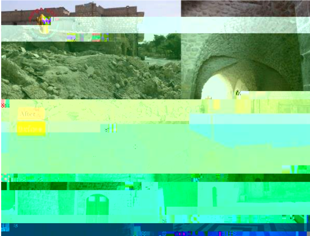
Damage to courtyard of al-Tawba Mosque, facing south, and 'before' photographs of interior (APSA; October 6, 2016)
