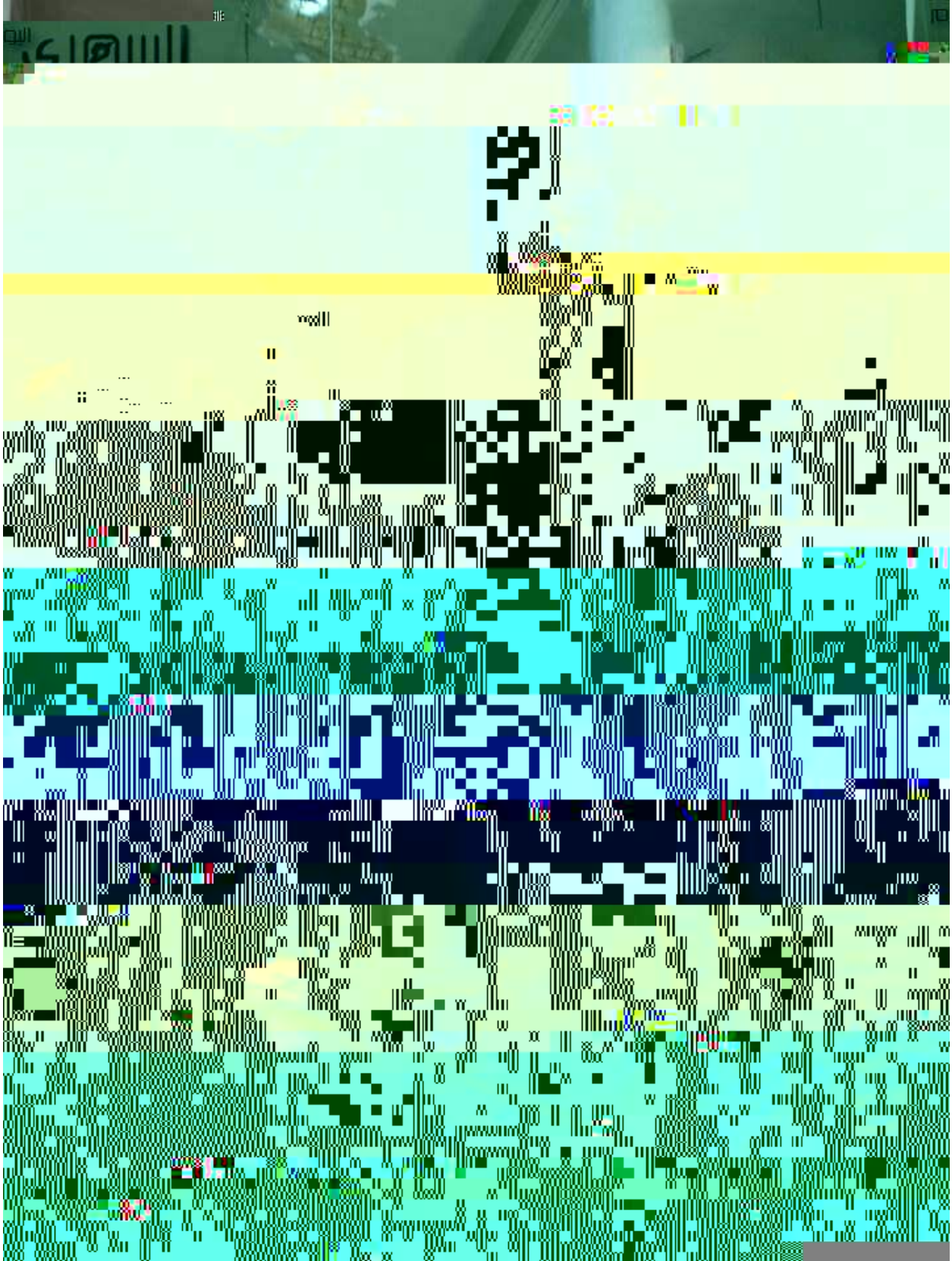
Damage to the interior of Saint Paul the Apostle Church (ASoury; September 5, 2016)
