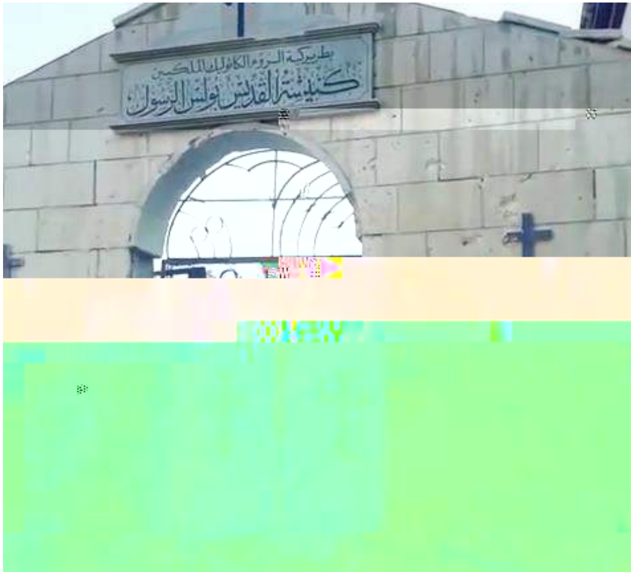
Video still of the damage to Saint Paul the Apostle Church (Today in Syria; August 26, 2016)
